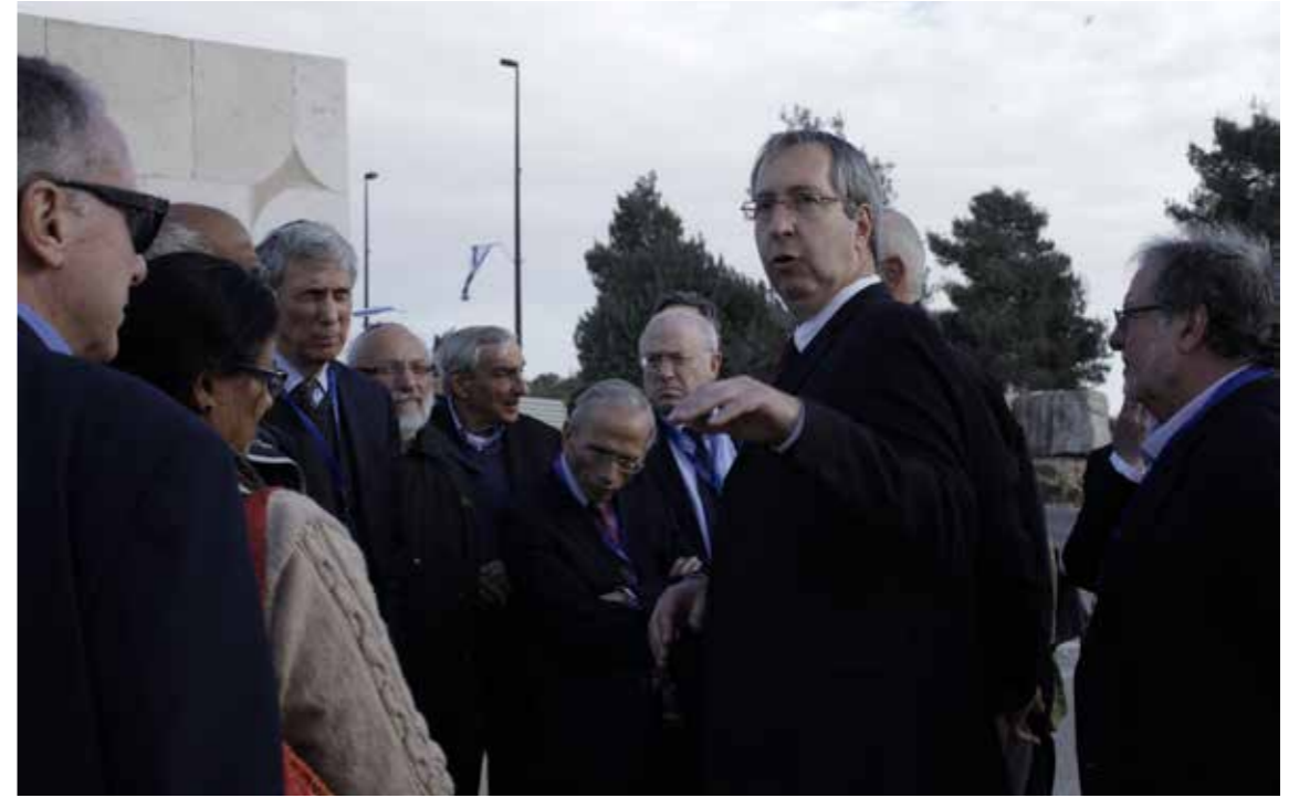
Global Forum members visit the building site of the New National Library of Israel complex.
